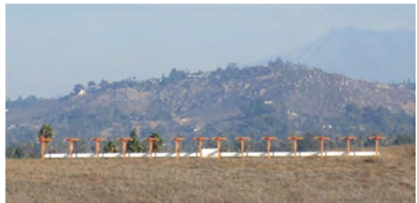
Localizer Antenna Array Serving Runway 9
